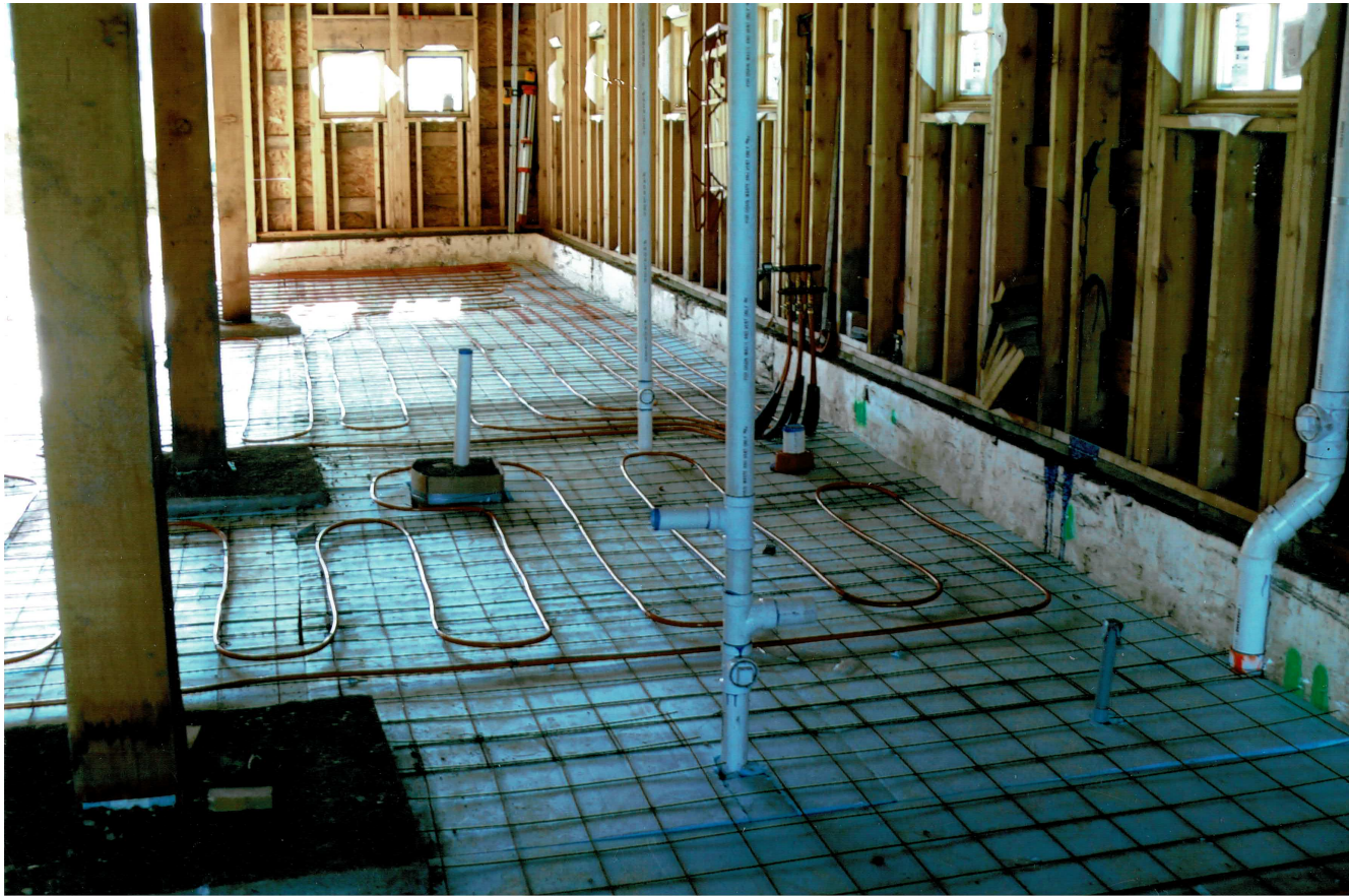
PHOTO SHOWS IN-FLOOR RADIANT HEAT INSTALLATION AT LOWER LEVEL. HOME HAS BOTH RADIANT HEAT AND FURNACE.
