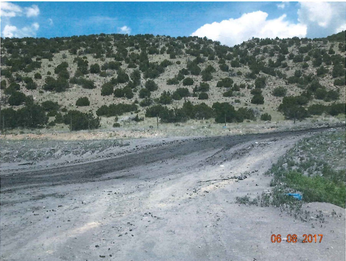
Photo 24: The fly ash-covered road near the Facility's solidification basin. Looking north.
